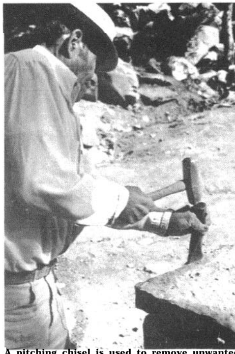
A pitching chisel is used to remove unwanted material in a hurry. Here Soto uses one to clean up a ragged edge on a flagstone.
